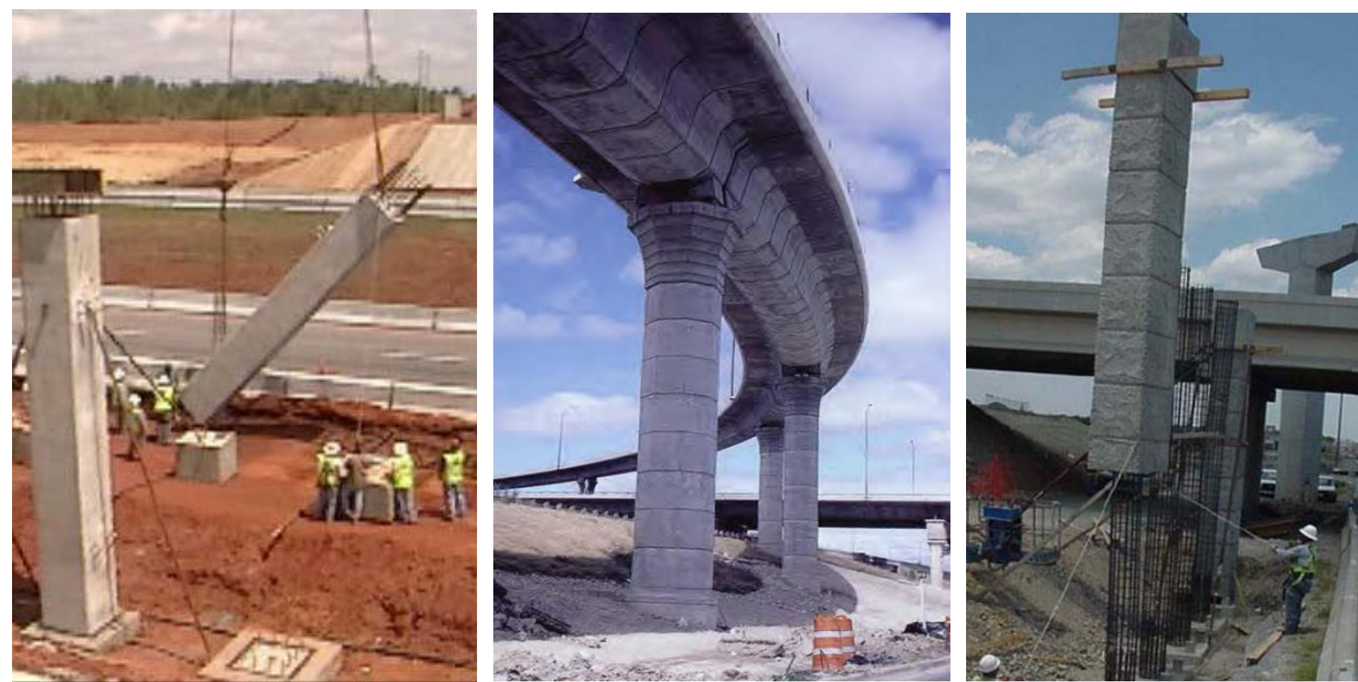
(a) full-height precast column (b) precast segmental column (c) precast column shell
